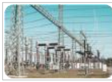
Power operation and maintenance
